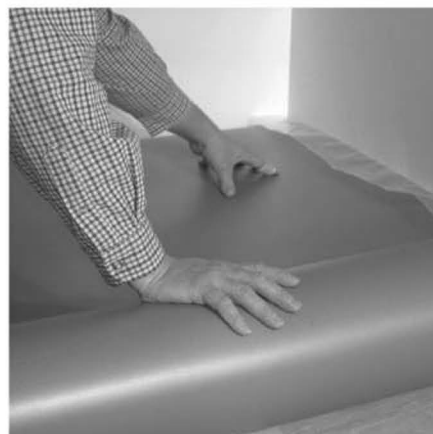
3. Roll out the underlayment, a few rows at a time to prevent tearing.
