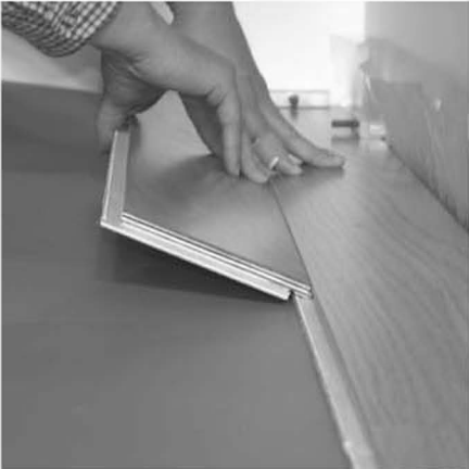
11. Position second row board at an angle and push down into place.
